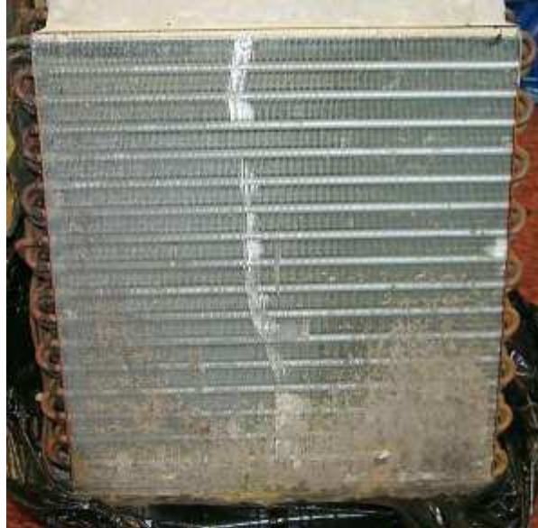
Buildup of mold biofilm in lower right hand corner completely blocks air flow
